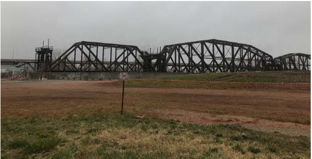
Figure 4. Site Photograph of the Rock Island Bridge looking southwest from 200 South James Street (provided by Planning Staff).
